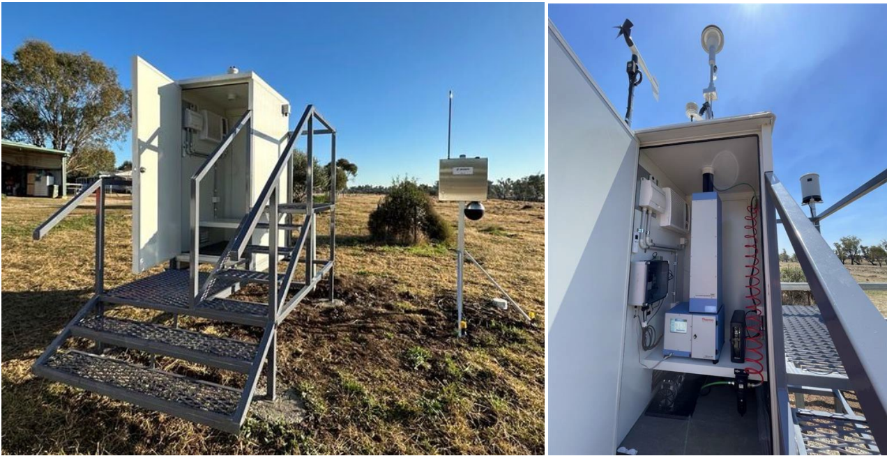
Figure 1: TEOM and blast monitor installed at Lanreef
